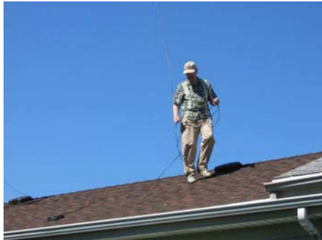
Fiddler on the roof Howard AK9F performs rooftop acrobatics while he erects the 40 meter antenna
